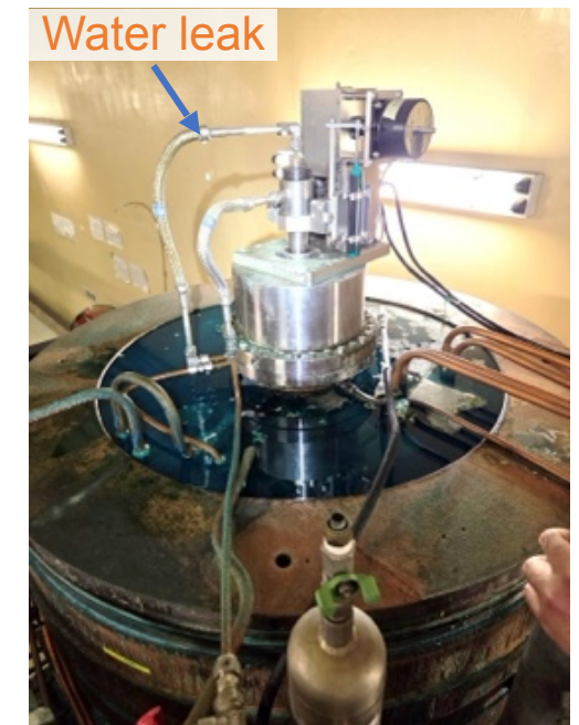
Cooling water leak at D05F cavity
