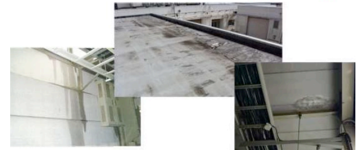
Water leak of MR power supply building
