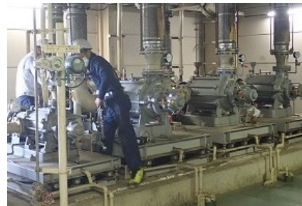
Water pumps at Fuji
