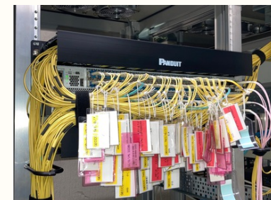
Core network switches
