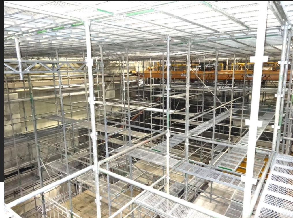
Scaffold to clean up walls and ceiling at acc. structure assembly room
