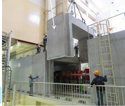
Concrete radiation shield
