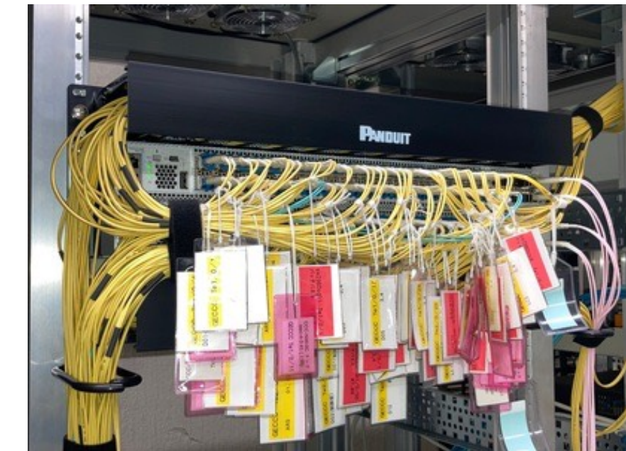
Core network switches
