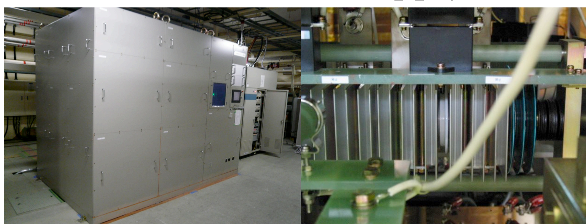
Picture of the power supply at the Linac Klystron gallery
