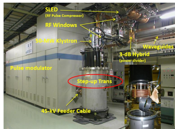
Figure 3: The linac damage in klystron gallery.
