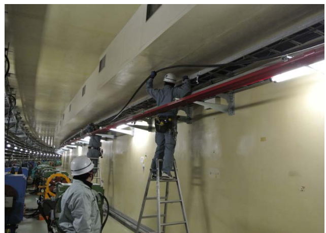
Figure6: LCX installation into the KEKB tunnel arc section.
