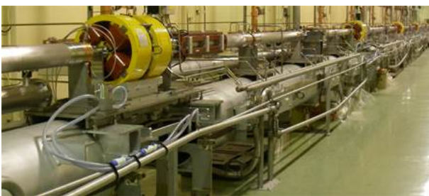
Figure 14: Hydrostatic leveling system.
