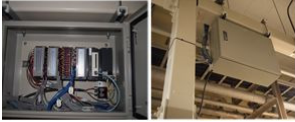
Figure 2: Picture of the data logger provided with the communication unit, power supply unit and input units.
