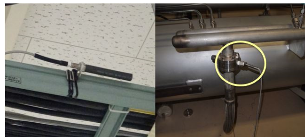
Figure 1: Pictures of the temperature sensor in the klystron gallery (left) and for the cooling water of accelerating structure (right).
