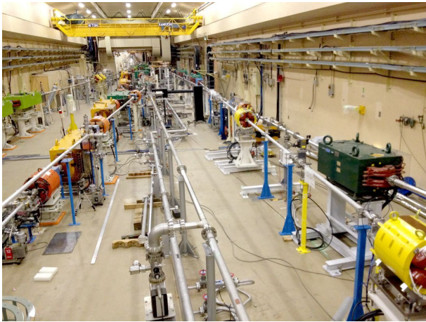
Figure 5: The beam switch yard at the end of linac. From right to left, beamlines of PF, PF-AR, straight dump, SuperKEKB LER, HER, and east dump.
