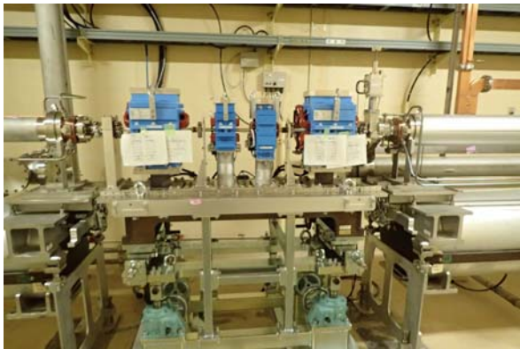
Figure 5: Photograph of the newly installed pulsed steering and quadrupole magnets.
