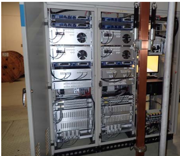
Figure 6: Photograph of the pulsed steering and quadrupole magnet power supply and control system. The control system is based on the PXI and CompactRIO buses. The control software comprises NI LabVIEW and EPICS frameworks.
