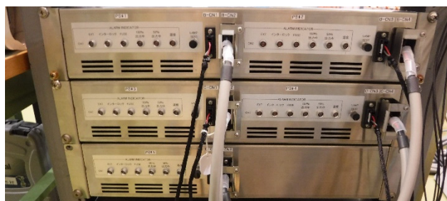
Figure 5: Photographs of the inverter units with the cooling fan.
