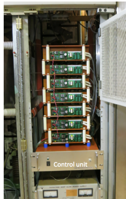
Figure 3: Solid-state thyatron replacement switch installed in modulator.
