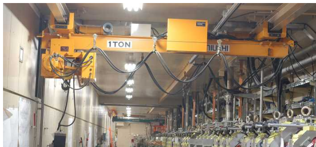
Figure 1: The crane at old positron source.
