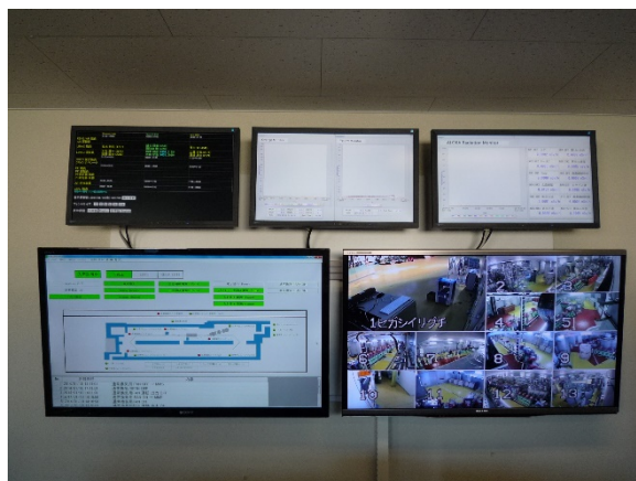
Photo 9: Monitors in the control room.
