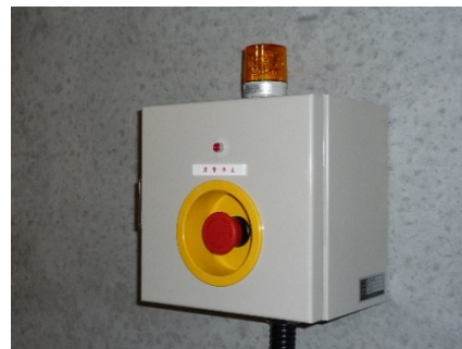
Photo 3: Emergency button (with a revolving warning light).
