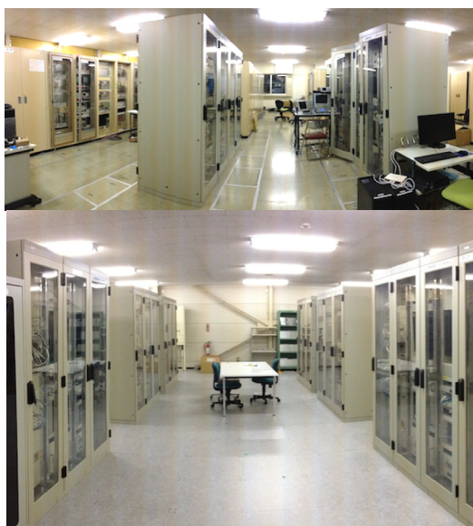
Figure 4: Installation appearance of new LLRF control systems in the RF control rooms of D4 (upper) and D5 (lower) section.
