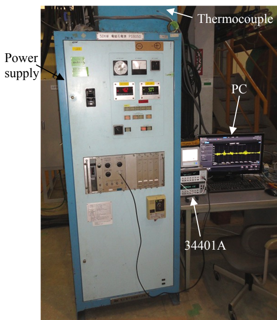
Figure 4: Photograph of power supply and measurement devices.
