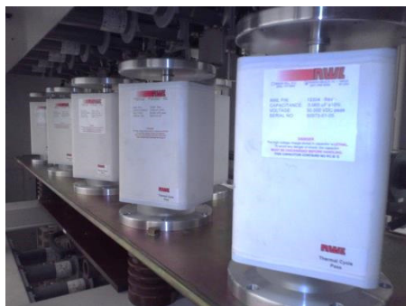
Figure 5: Photograph of new capacitors installed in PFN with specially designed attachments.
