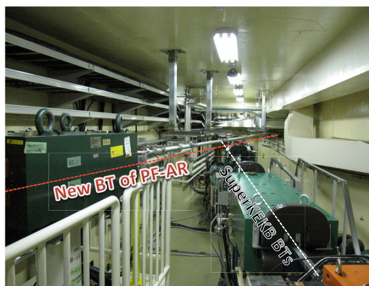
Figure 6: Three 4 m-long vacuum ducts for the new BT of PF-AR were hung on the ceiling of the existing SuperKEKB BTs tunnel.
