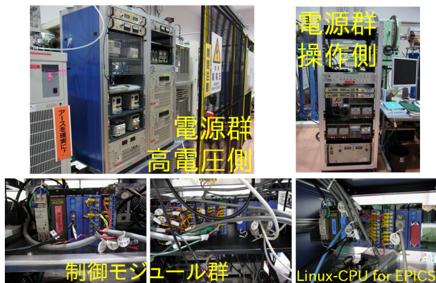
Figure 3: PIS power supply and control system hardware.
