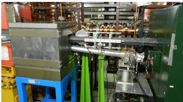
Figure 7: Abort beam position monitor in front of the beam dump.
