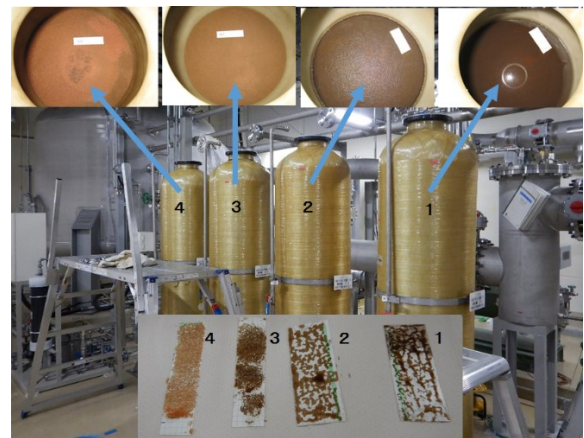
Figure 2: Contamination of RI4 water flow system.
