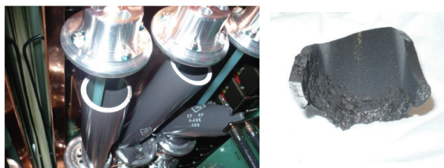
Figure 3: Broken ceramic resistors connected with the shunt-diode.
