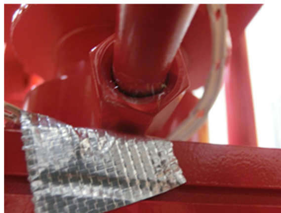
Figure 4: Leakage of Cooling Water from the Connector of No.2 Mod. Klystron.
