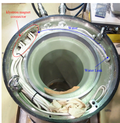
Figure 6: Klystron magnet water leak point.
