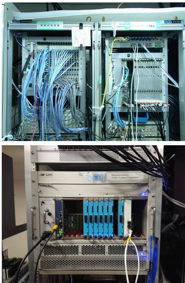
Figure 2: (Top) old and (bottom) new LLRF control systems.
