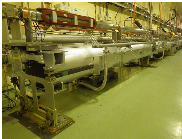
Figure 1: Standard accelerator girder at LINAC.
