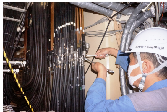
Figure 5: Picture of replacing the water-cooling hoses of the cyclotron main coil.
