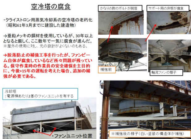
Figure 9: AFC severely damaged by corrosion.
