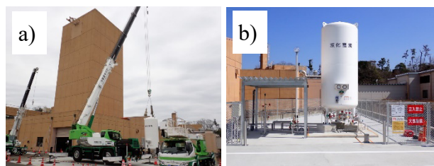
Figure 2: a) Photo of construction work of cold evaporator (CE) of liquid nitrogen. b) Completed CE.
