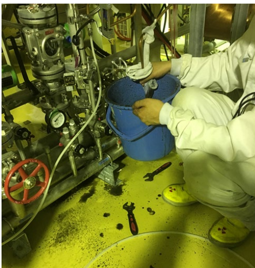
Figure 1: Inquiry into contamination of water cooling system.
