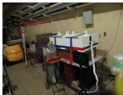
Figure 6: The beam dump at the end of injector linac.
